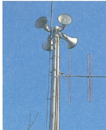
Disaster Prevention Wireless Towers
